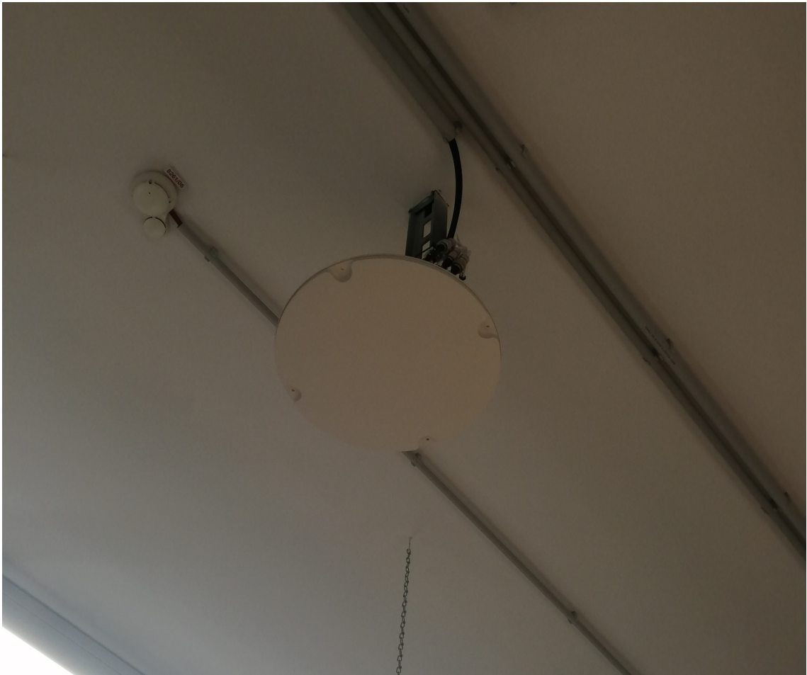
Figure D.1: 5G Antenna at Gateway Gründungsservice (bottom view)
