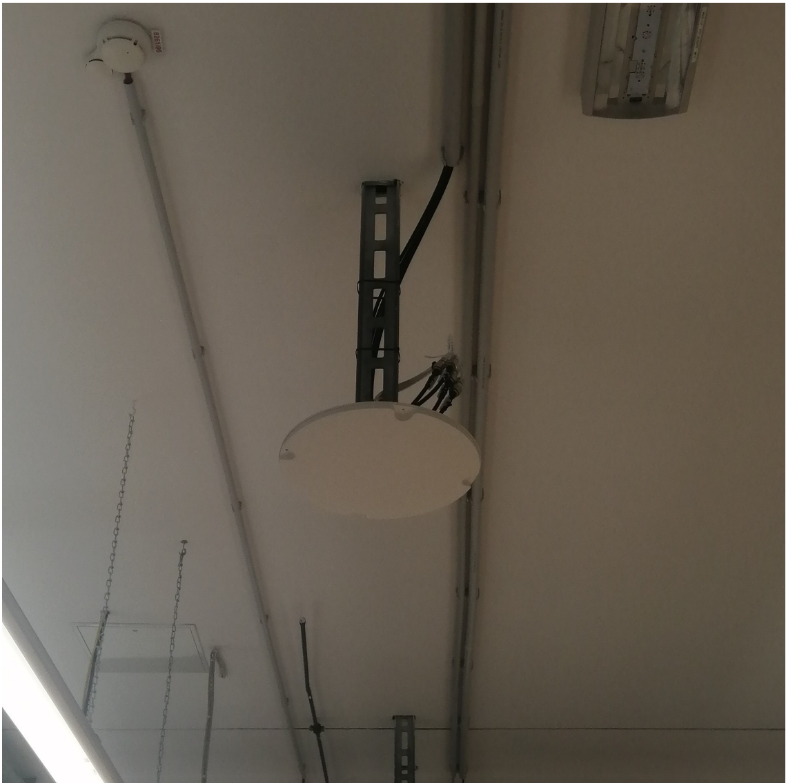
Figure 4.6: 5G Antenna at Gateway Gründungsservice (side view)
